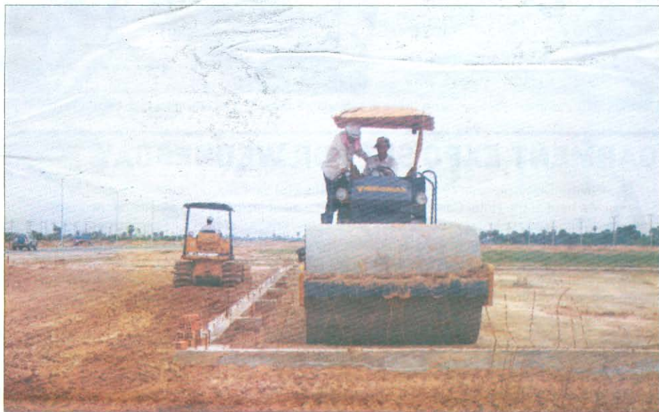
Workers prep the site of the Phnom Penh SEZ in this file photo. BY KAY KIMSONG
